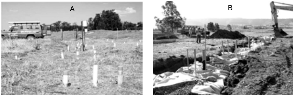
Figure 6. (A) Pilot-scale PRB with piezometers and monitoring wells in ASS terrain on Shoalhaven Floodplain, southeast NSW and (B) installation of the PRB
