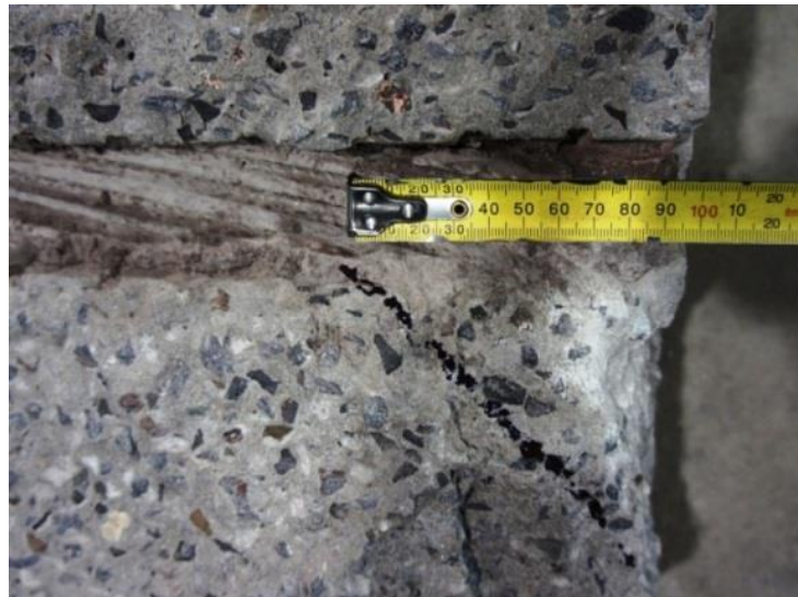
Figure 8: Cable bolt deflection
