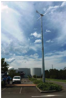
Figure 8 Aerogenesis 5kW wind turbine. One of two to be used to power the SBRC building, mounted on 18m articulated towers.
