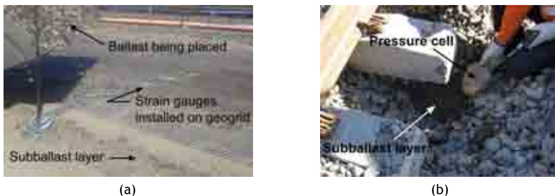
Figure 5: Installation of (a) strain gauges and (b) pressure cells to monitor response of track substructure under repetitive wheel loads.
