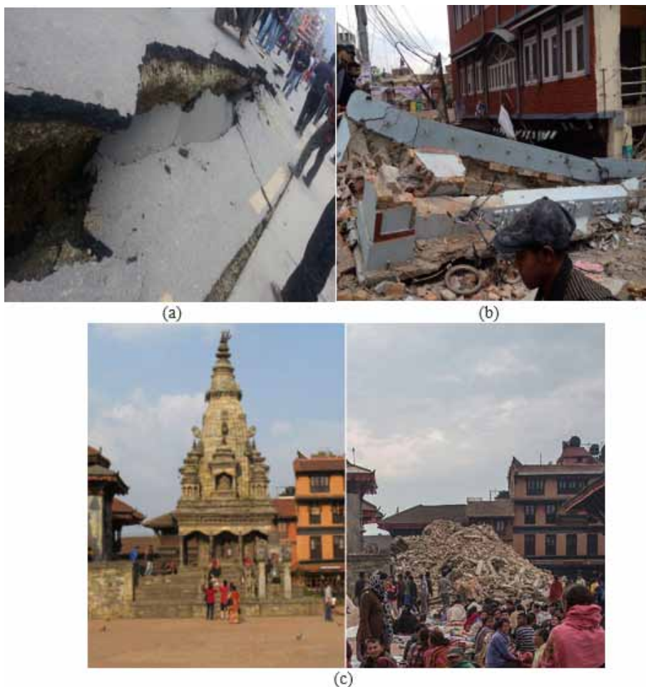
Figure 6. Some structural damages in Kathmandu during 2015 Nepal earthquake of Mw 7.8 (after https://images.google.com ) (a) Collapse road (b) collapsed building (c) Collapsed temple
