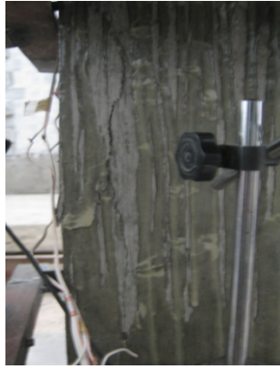
(a) Vertical crack near column corner
