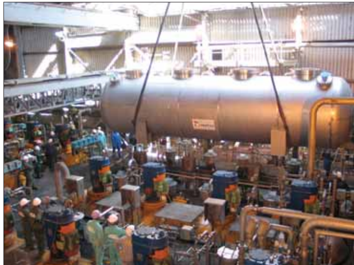
Figure 10—Installation of the completed second stage leach autoclave at the BMR in June 2007
