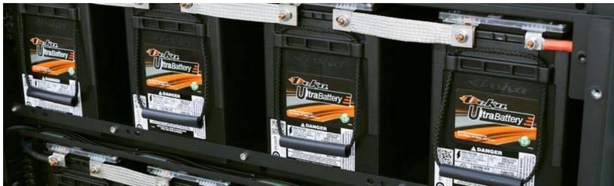
Ecoult Ultrabatteries photographed during installation on site. from www.ecoult.com
