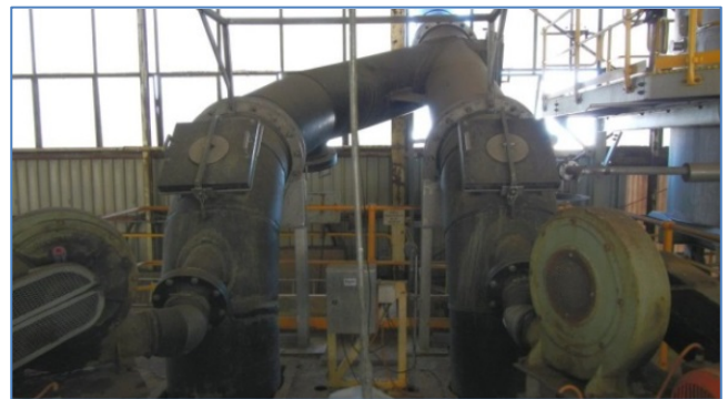
Image 1: Purification tank extraction system (Roseberg 2015)
