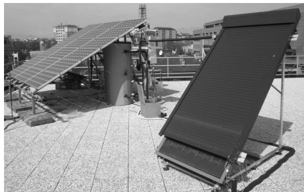
Figure 1. The PCS-based solar thermal system prototype.
