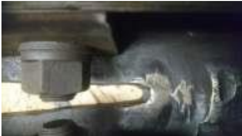
Photo 3 – Fracture site in rail convergence.
