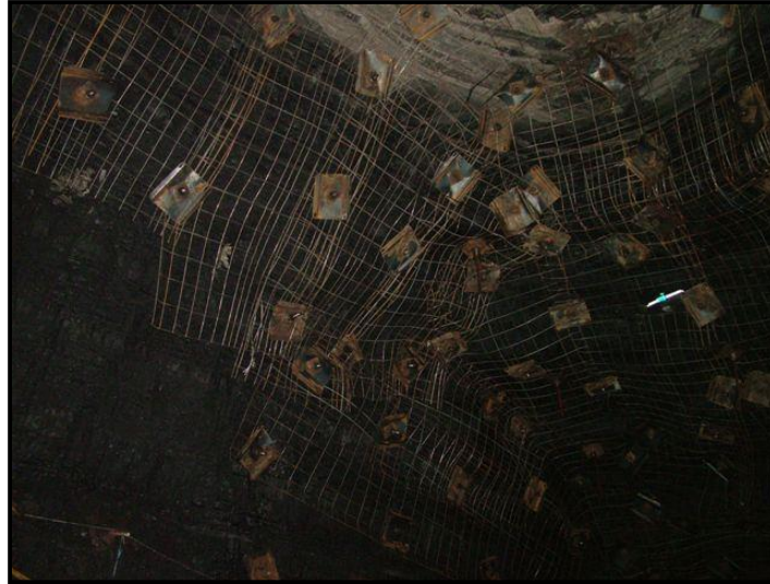
Figure 3: A rib with intersecting structures and roof cavity showing coverage provided by bolts and mesh.
