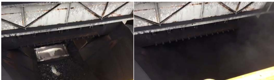
Figure 4: Dust escaping through opening for feeder
