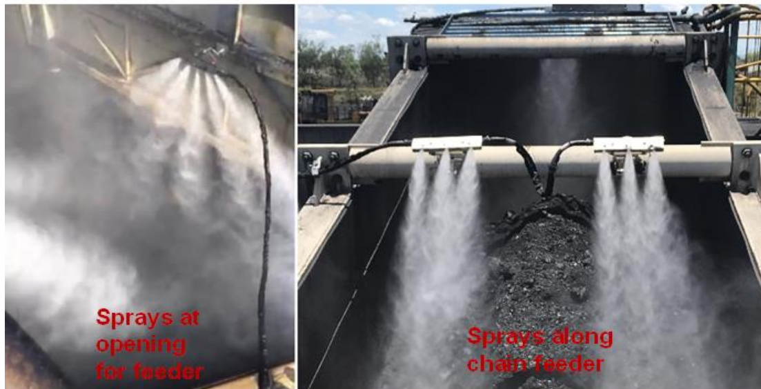
Figure 6: Installed dust suppression system at exit of hopper, along chain feeder and at transfer from chain feeder to primary sizer
