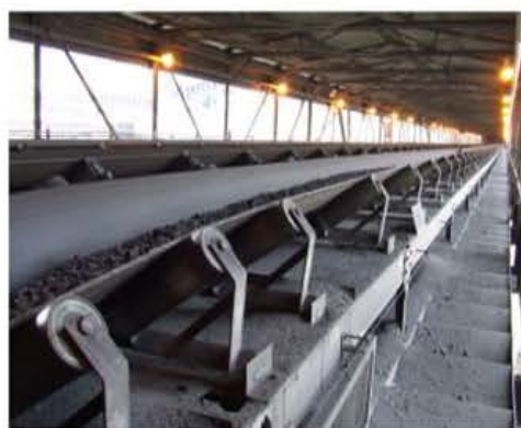
Figure 3: Inclined Conveyor from Coal Bunker
