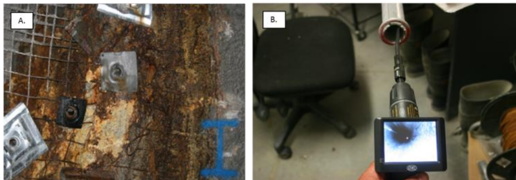
Figure 12: Observed corrosion of existing galvanized ground support through surface and penetrating visual means at Mine B
