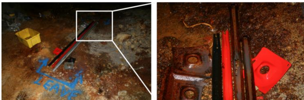
Figure 13: Observed corrosion of Enduro™ (black) and (red-bolt) at Mine B
