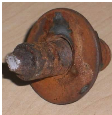
Figure 1: Corroded and failed roof bolt
