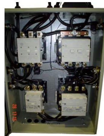
Figure 6. Test System Contactor Enclosure
