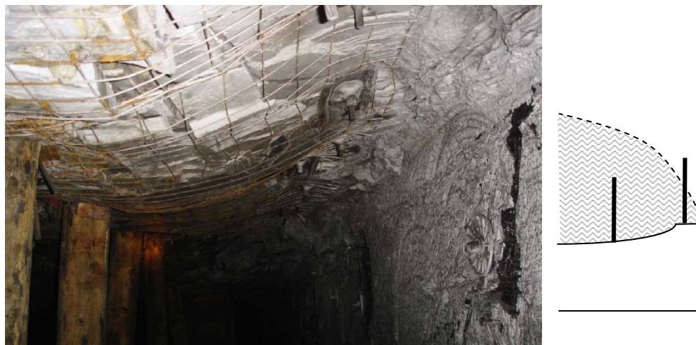
Figure 14 - Common roof deformation pattern is consistent with outer bolts being the only ones anchored
