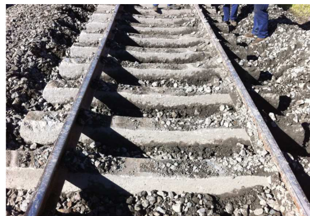
c) fouled/crushed ballast, abrasion of sleeper soffit and overstressed formation (after excavation)
