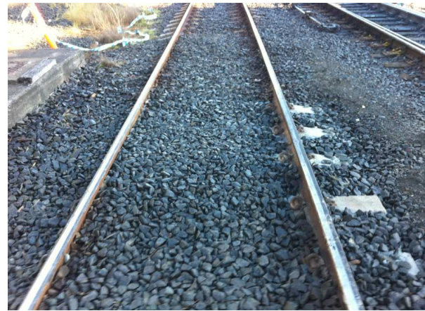
a) deteriorated track (large localised settlement)
