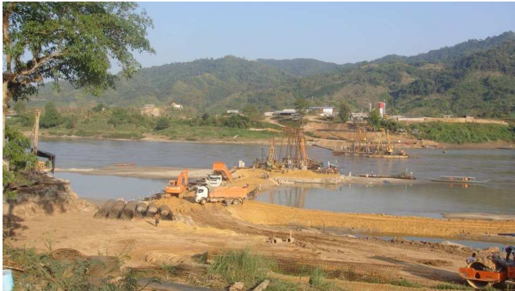
Figure 3 here, Caption: Constructing a Bridge, Completing the Corridor (January 2012) 338x190mm (72 x 72 DPI)
