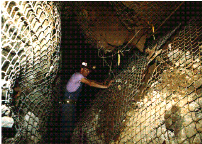
Fig. 1 Damage to a drive from rockburst
