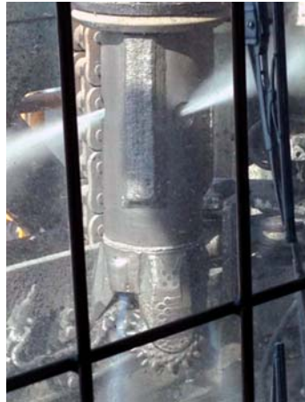
Figure 2: Water spray from weep holes in side of the sub above the drill bit
