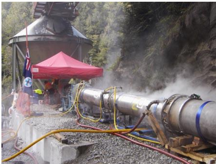
Figure 3 - The GAG jet inertisation system in operation at Pike River (NZ Police, 2012)
