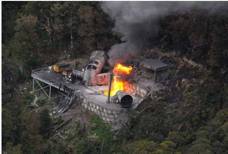
Figure 2 - Fire burning at top of fan shaft after fourth explosion (NZ Police, 2012)
