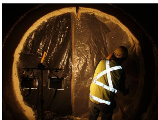
Figure 6 - Plastic curtain to seal gas volume
