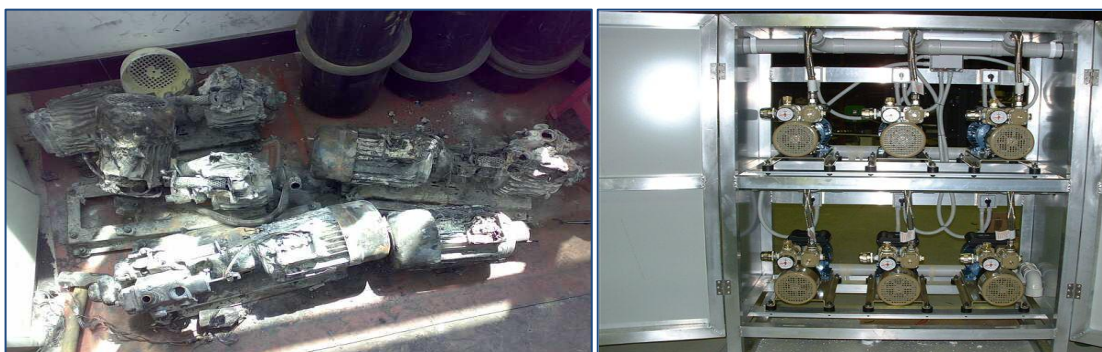
Figure 1 - An example of damage to a tube bundle pump system located on the surface
