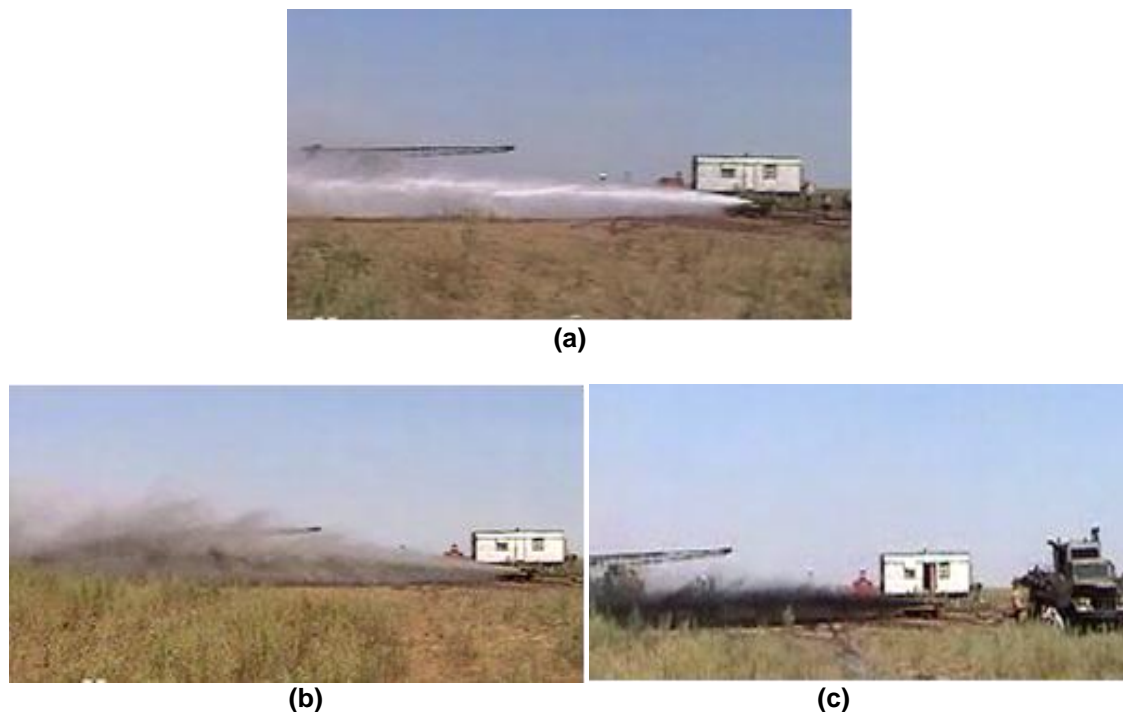
Figure 1 - Coal fines plug being cleared from hole, shown as a black jet flowing from the borehole as it is opened up after hydrofrac-pumping
