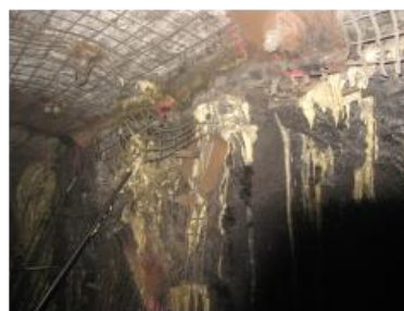
Figure 7- PUR injection of upper rib Mudstone interbedded with coal lenses
