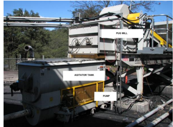
Figure 5 - Field trial plant
