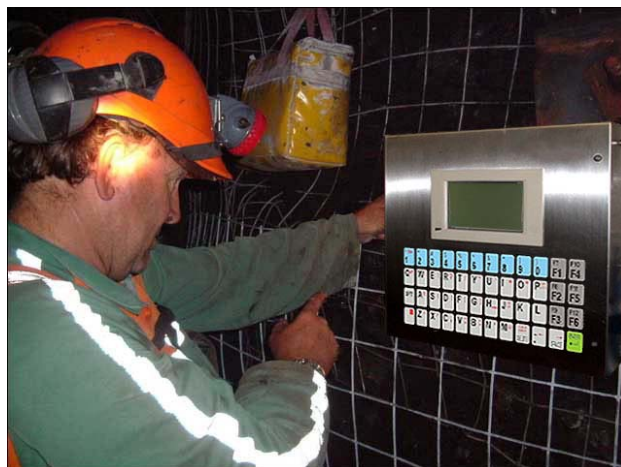
Figure 3 - Depiction of the proposed low-power email/messaging device. It is envisaged that the device would be powered via a small number of fibre optic cores.
