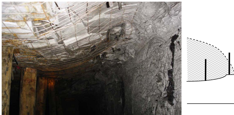
Figure 14 - Common roof deformation pattern is consistent with outer bolts being the only ones anchored
