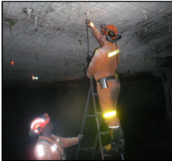
Figure 3 - Photo showing transducer (vertical) held at the end of bolt (i.e. collar of hole) at Manadalong Coal Mine
