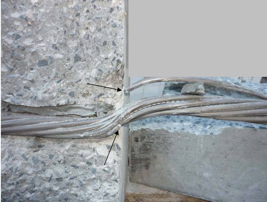
Figure 8 - One element failure on the LHS sheared plane face
