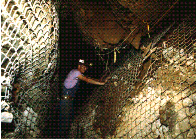
Fig. 1 Damage to a drive from rockburst
