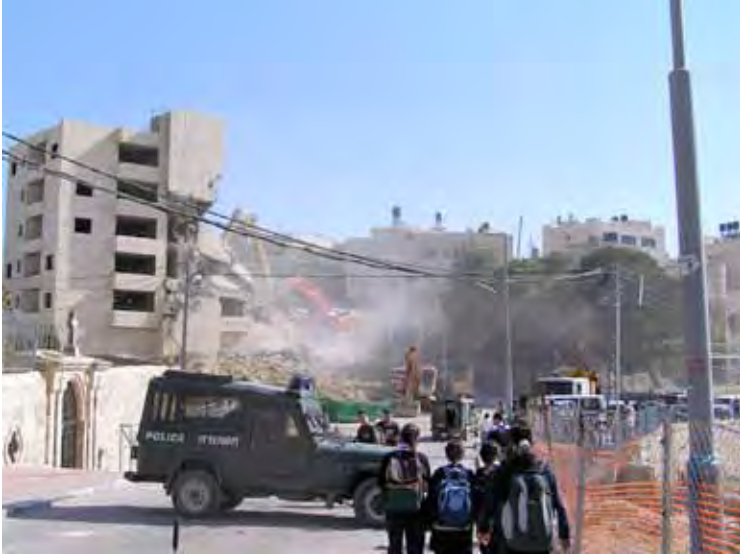
Demolition of Palestinian homes by Israeli authorities. Photograph by Jennifer Killen, February 2005.
