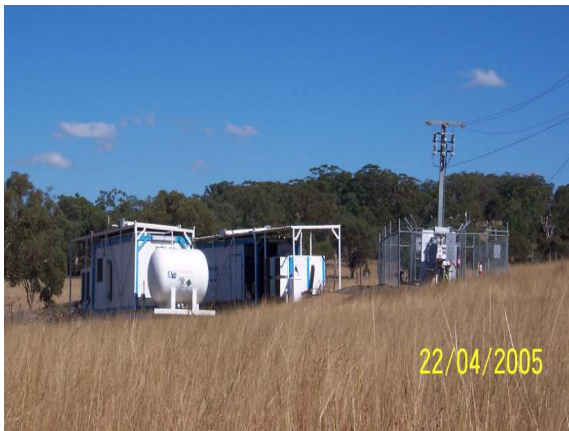
Figure 6 - "AMSA" Membrane filter at a Hunter Valley Coal Mine
