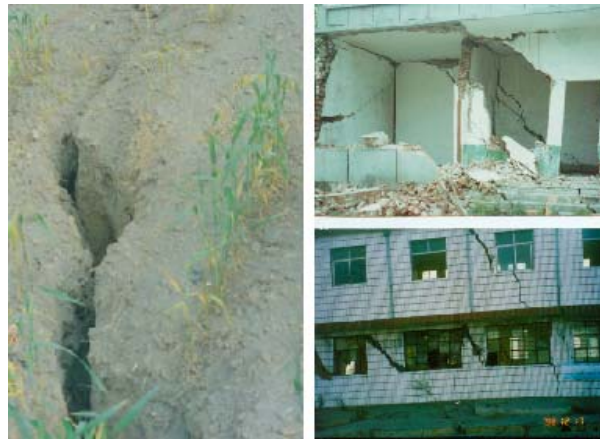
Figure 2 - Farmland and structures damaged by mining
