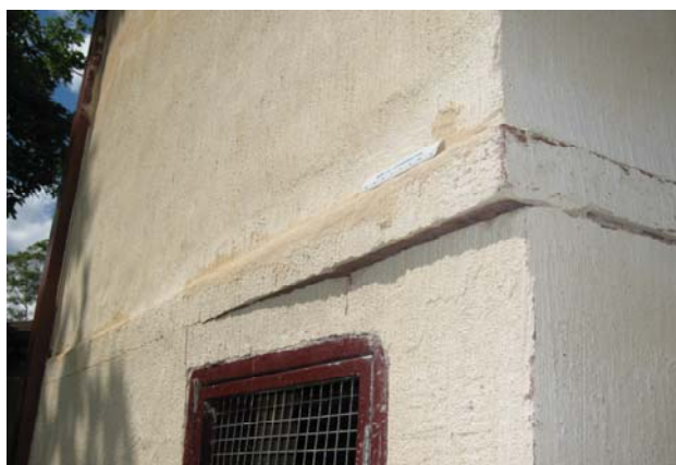
Figure 1 - Structures Affected by Horizontal Shear Deformations
