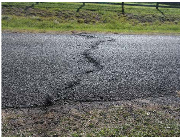
Figure 3 - Mining-induced surface wrinkles
